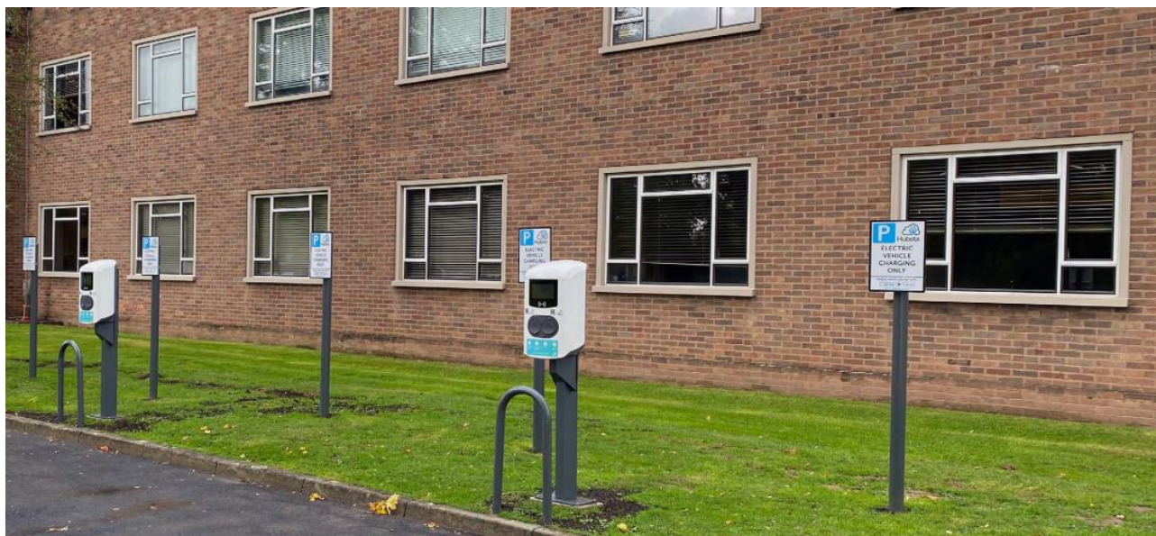
Figure 13: EA Technology Workplace Charging Installation 14
